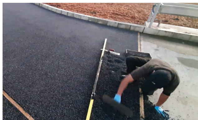
Experimental pour-in-place rubber surface prior to adhesion of a geotextile top surface.
