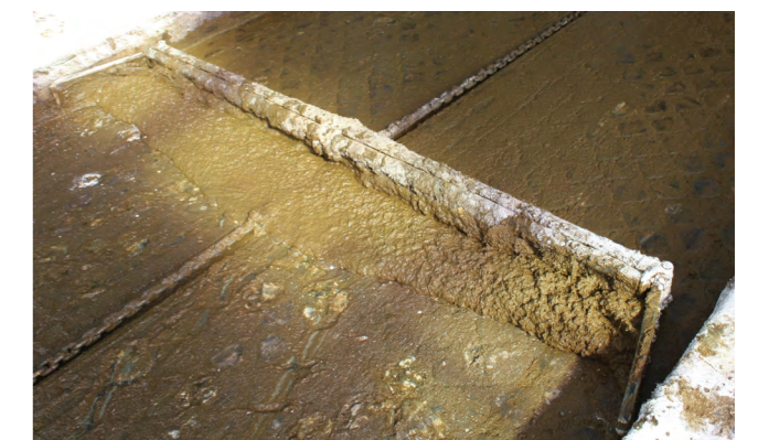
Ensure the scraper runs frequently enough to keep the volume of scraped slurry from overflowing onto the beds.
