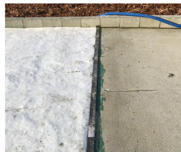
Flood wash risers imbedded in the concrete. Water flows from right to left.
